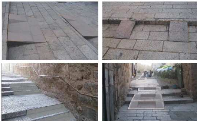
Examples of implementation of an extended continuous ramp, based on existing conditions and their completion into a single unit of minimum dimensions.
