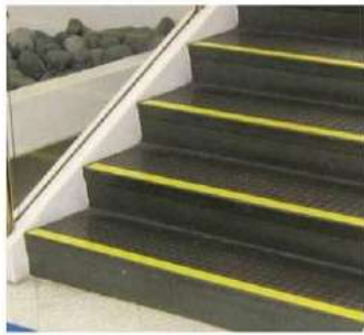
External stairs with painted leading edge
