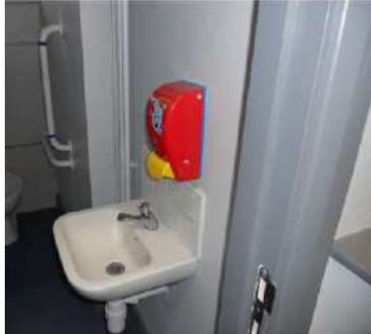
Soap dispenser contrast. Handrail & Sink could contrast better from wall
