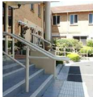
Poor Handrail design
