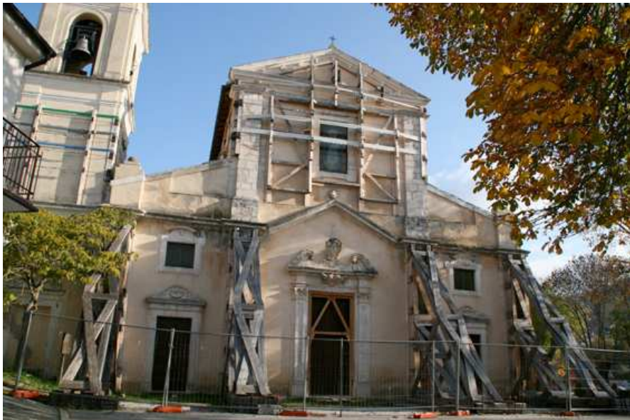
Photo 3 Goriano Sicoli, the Church of St Gemma after the earthquake.
