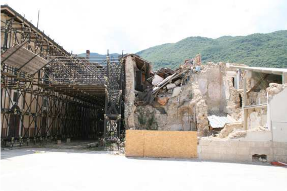
Photo 1 The destruction caused by the earthquake and propping and securing works in one of the small villages in the "earthquake crater".
