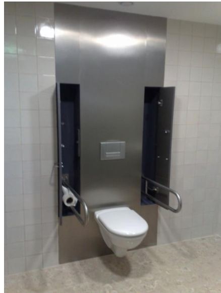
Figure 6: National Tile Museum, active assistance bars (Detail) (source ProAsolutions.pt Lda)
