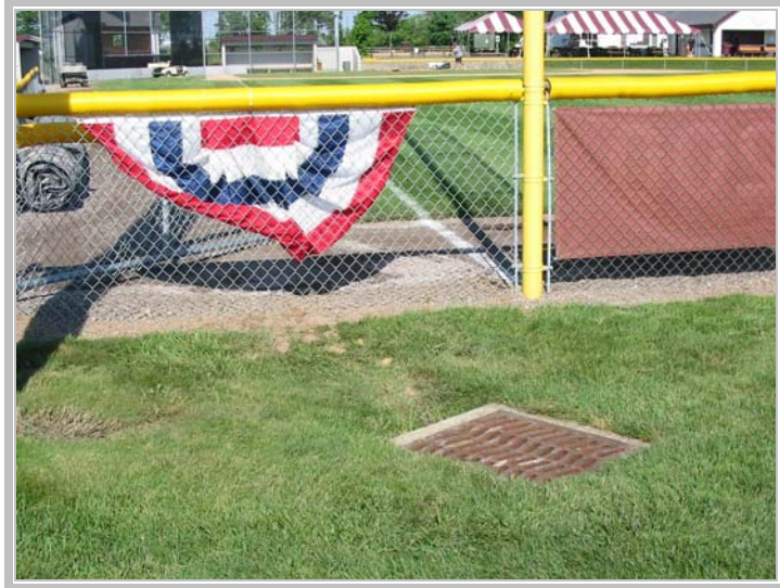
Figure1. Catch basins should be located outside the fences surrounding the playing area to prevent player injury.
