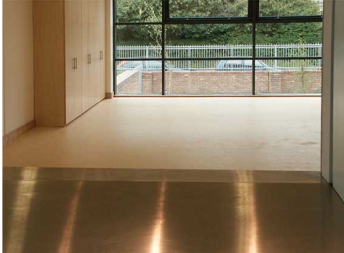
Fig 5. The change of surface and reflectivity in this circulation space causes most users to hesitate; "Is there a step here?"- in fact it is level.
