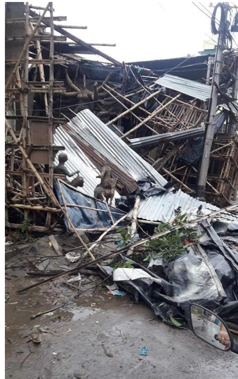
Figure 3 : Image showing the condition of the workshops after cyclones
