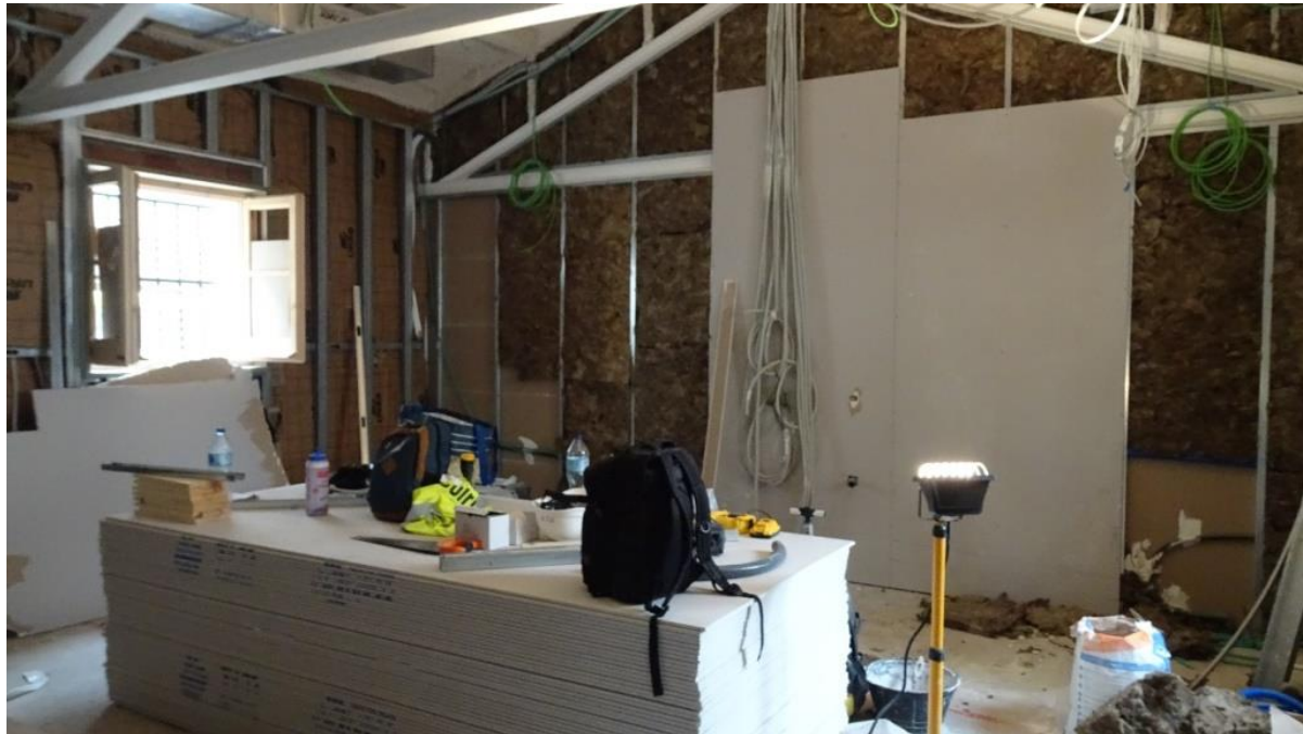
Figure 6b. Remodelling work on the old houses to convert them into a museum space (MUHBA) and headquarters of the Bon Pastor-Baró de Viver remembrance archive. The museum is expected to open in February 2023.
