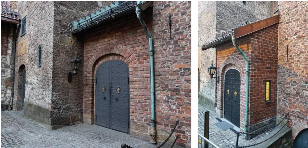
Figure 6. L.h.s.: The church's entrance hall before intervention. R.h.s.: The church's entrance hall after intervention. (Photo: Oslo Byggher AS)
