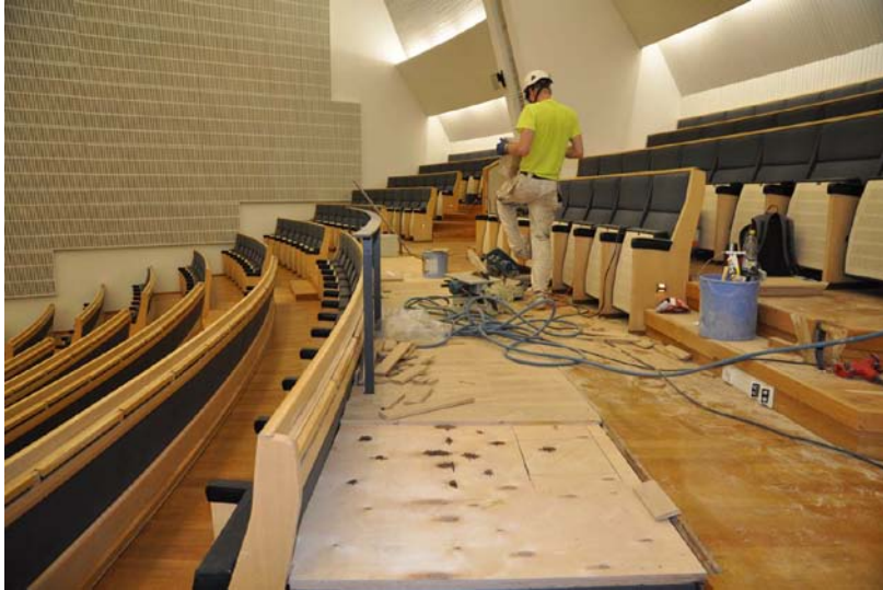
Figure 13. New seats for spectators using wheelchair were designed to hide well in existing seat rows of the Aalto Hall. Aalto University/Jarmo Tiirikainen.
